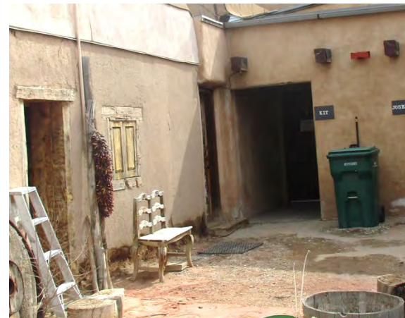
The Romero House wall by the bench on the left in this photo, the site of core sample #11, is constantly wet, consistent with site drainage issues noted in this area.
